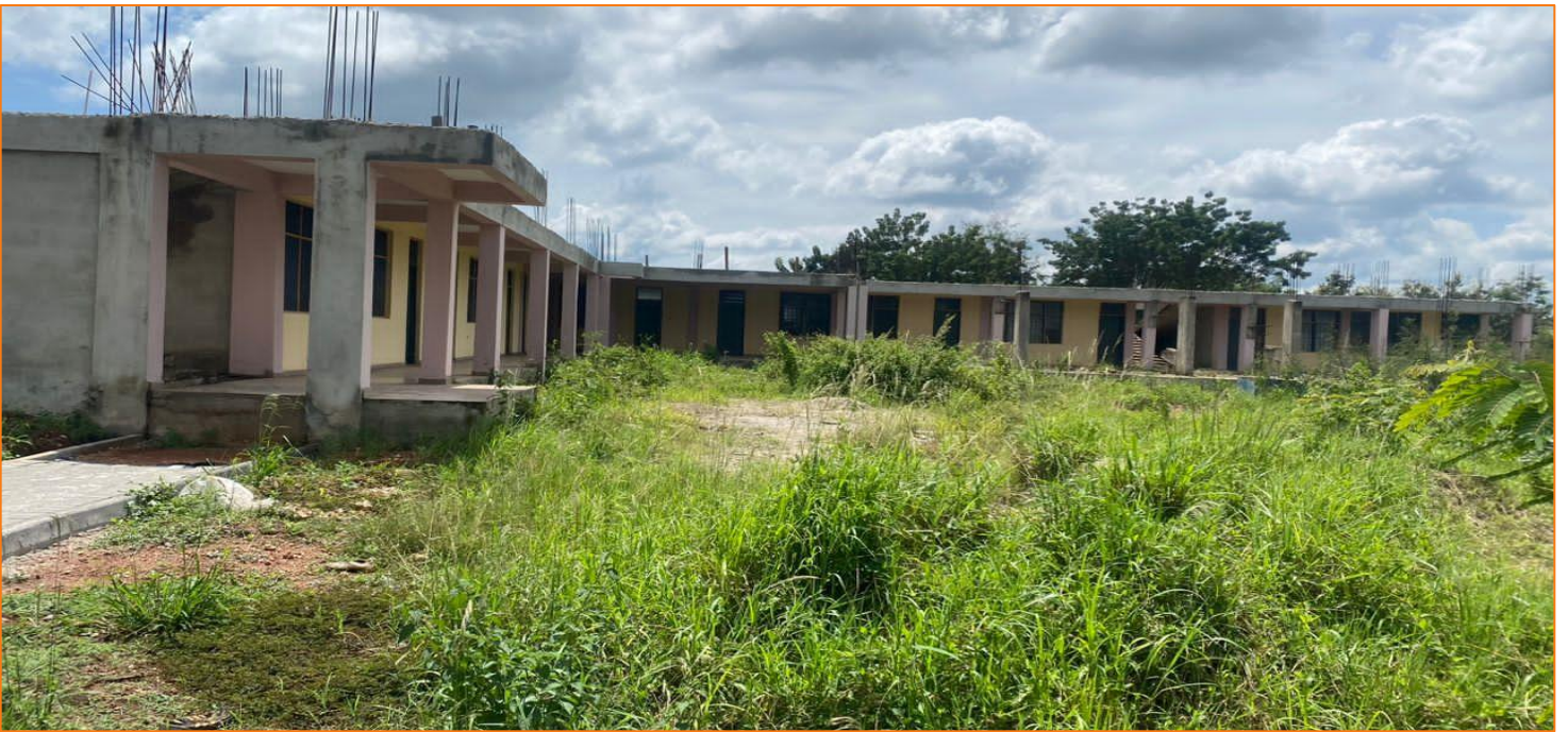
Constructed of 1no. Storey, 10units office complex block and external works at Berekum
