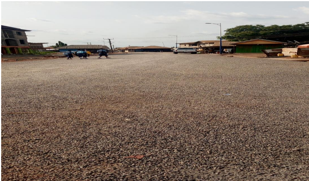
Tarred 243m road, installation of street lights, 1No. Traffic light and transformer
