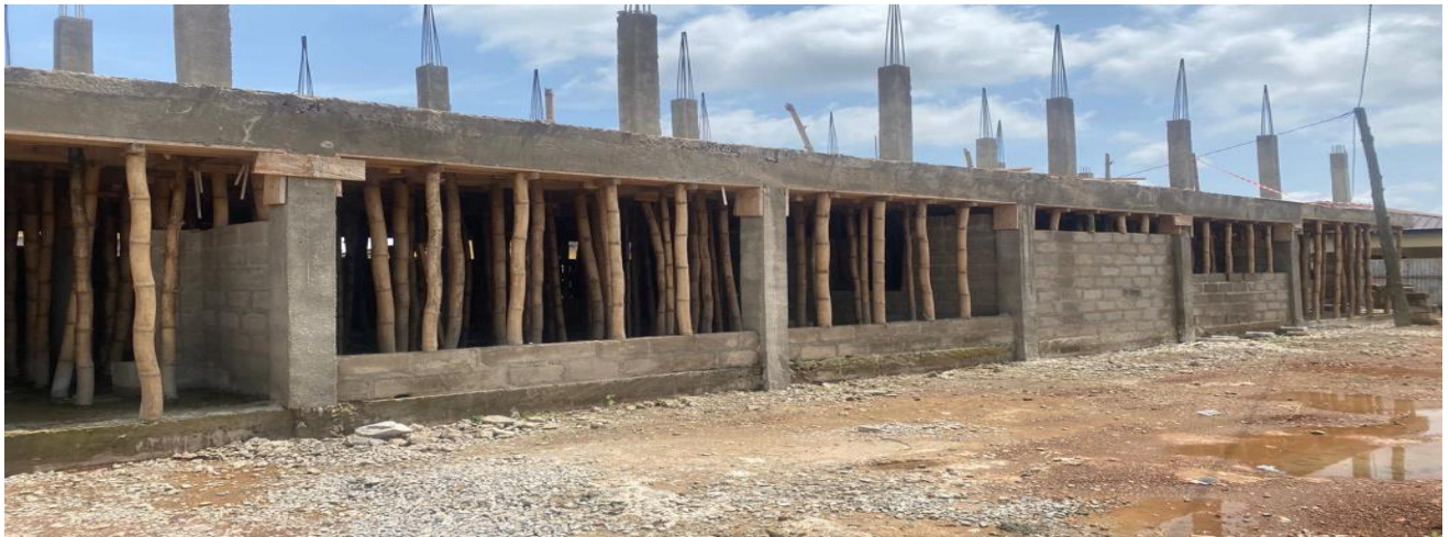
((Construction of 1No 40No. lockable stores, banking hall and external works at Berekum Thursday Market) - GSCSP
