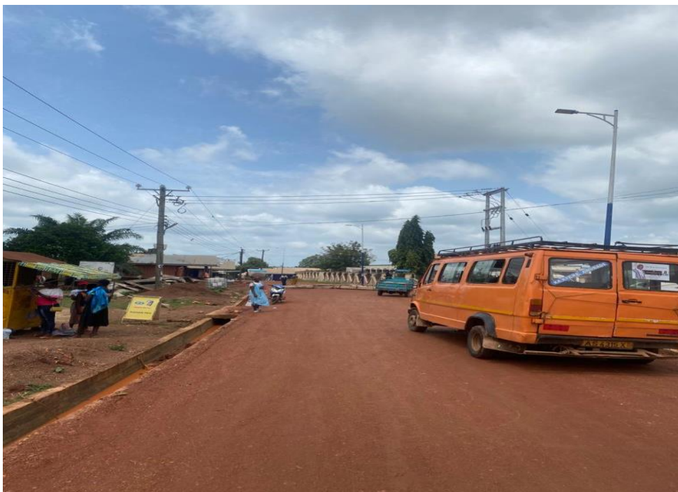
(Tarring of 243m road, installation of street lights, 1No. Traffic light and transformer at Berekum Thursday Market) - - GSCSP
