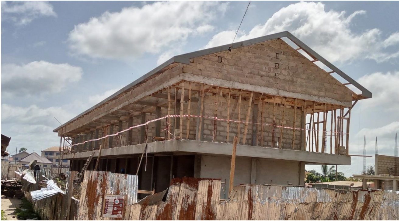
(Construction of 1No 48No. lockable stores and external works at Berekum Thursday Market) - GSCSP
