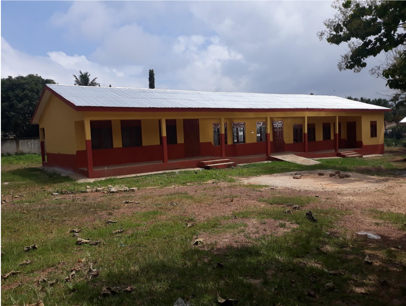
Figure 4. Construction of 1No. 3-Unit Classroom Block with ancillary facilities at Berekum RC Mixed School-Atonitia
